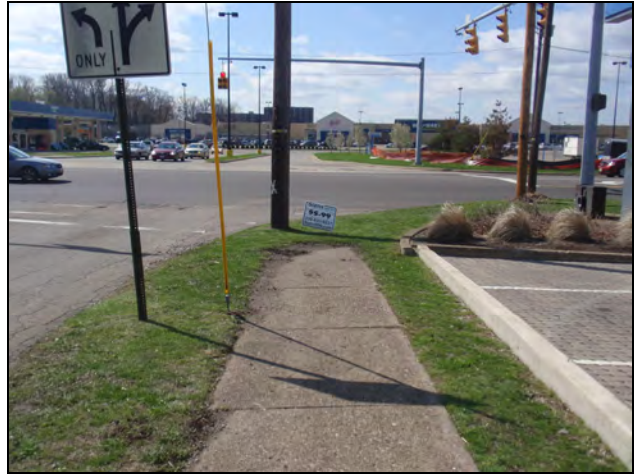
Incomplete Sidewalk at Intersection at Valleyview
